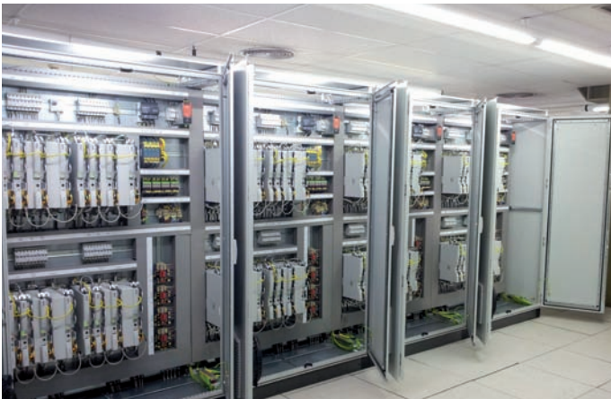
Servo Invert, Servo Takeout and Servo Pusher Control Cabinets.
