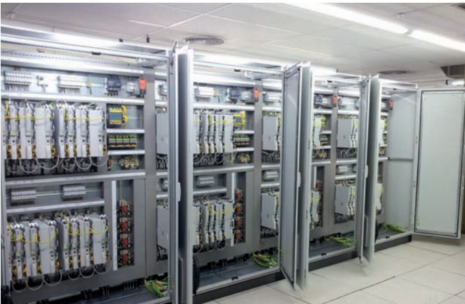
Servo Invert, Servo Takeout and Servo Pusher Control Cabinets.
